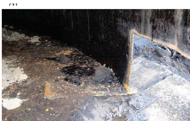
Fig.2. Corrosion faults of the lower belt and bottom in combination with the base setting. SVR 3000m 3 [3]
