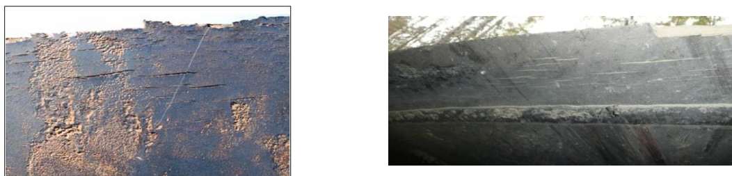
Fig. 1. Stress-corrosion crack on pipe-surface
